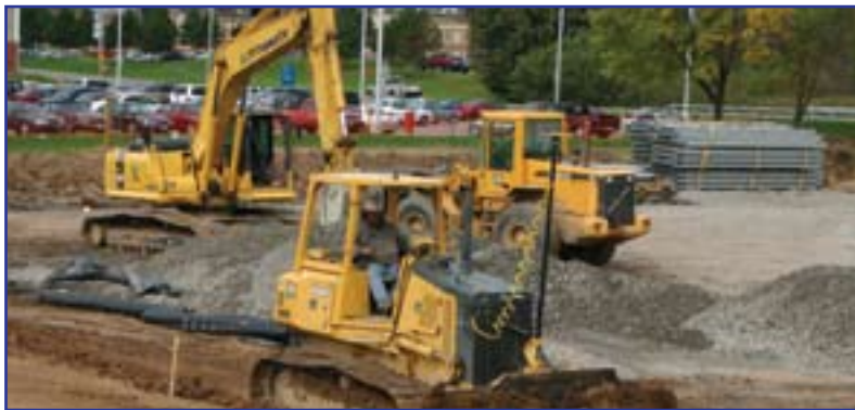
This project would be a first for DDS with the application of Global Positioning Satellite (GPS) technology on a dozer.
