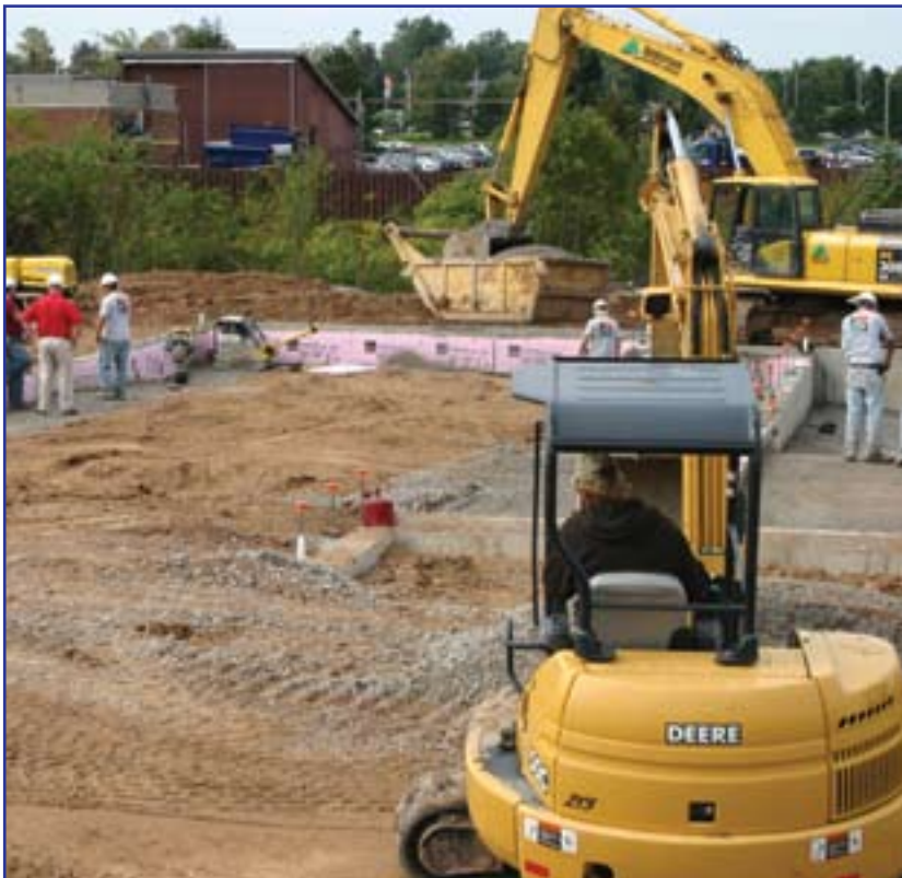
The excavation was then backfilled with suitable material and compacted in controlled lifts.
