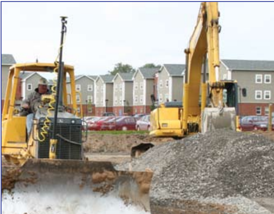
Poor soil conditions required substantial cut and fill for the size of the site. Approximately 20,000 cubic yards of material had to be excavated and exported.
